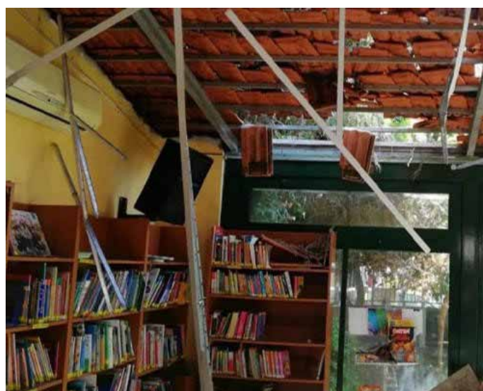
Effects of damage in Al-Sabeel library
